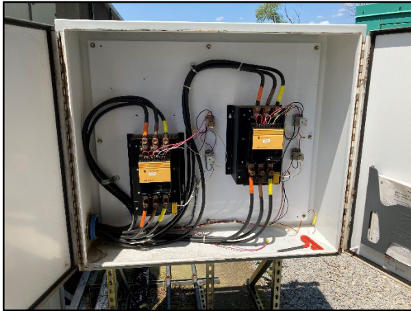
Soft Start Switches (A & B)
