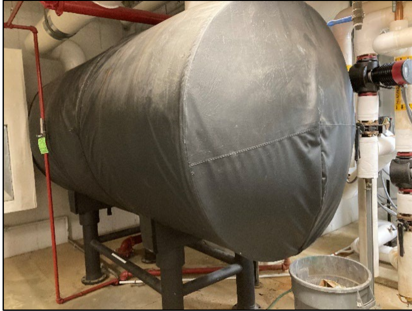
Chilled Water Storage Tank
