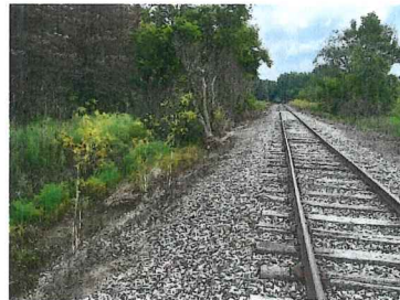
Left side of photo is east side of tracks (ditch). Right side is west side of tracks. No ditch was constructed along west side of tracks to help with drainage for Volkers #2.
