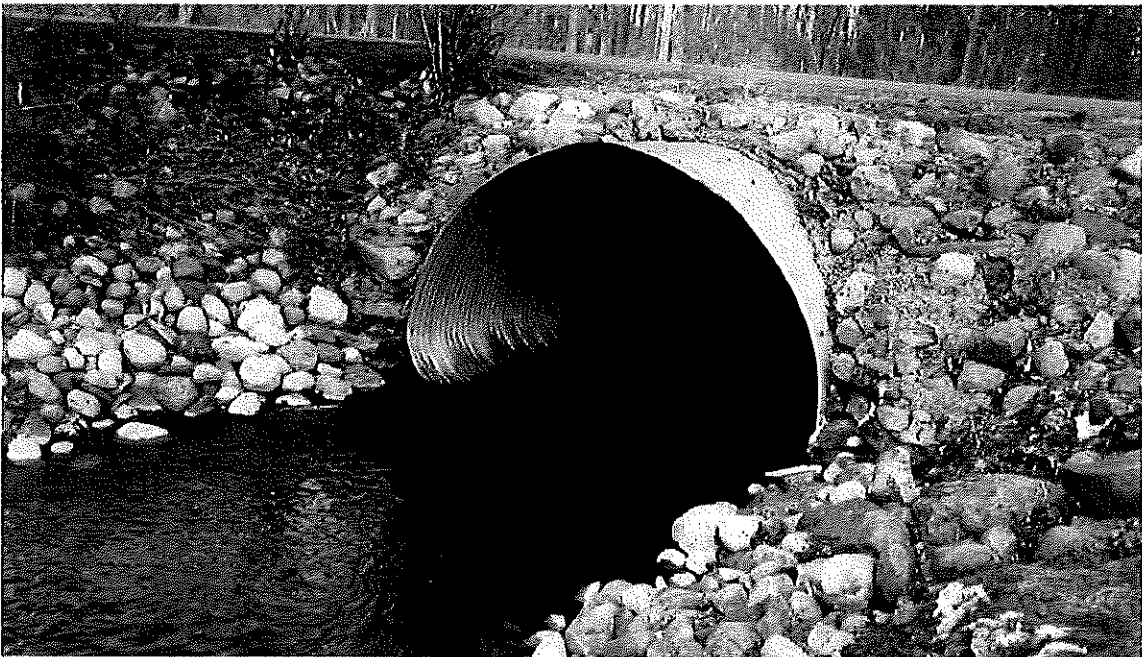
Picture No. 8 is the western upstream end of the 7.5-foot by 11.5 foot elliptical CSP culvert. There is slight distortion near the springline of the pipe. Picture is taken looking towards the northeast.
