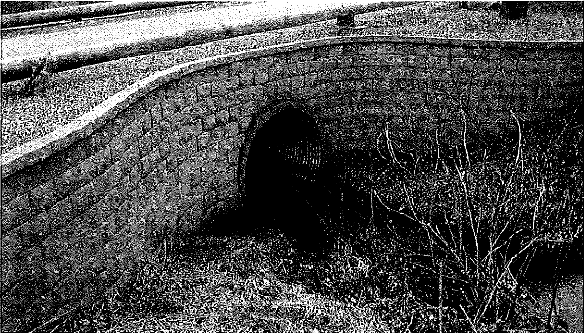
Picture No. 18 shows the western upstream end of the 66-inch CSP culvert. Picture is taken looking southeast.
