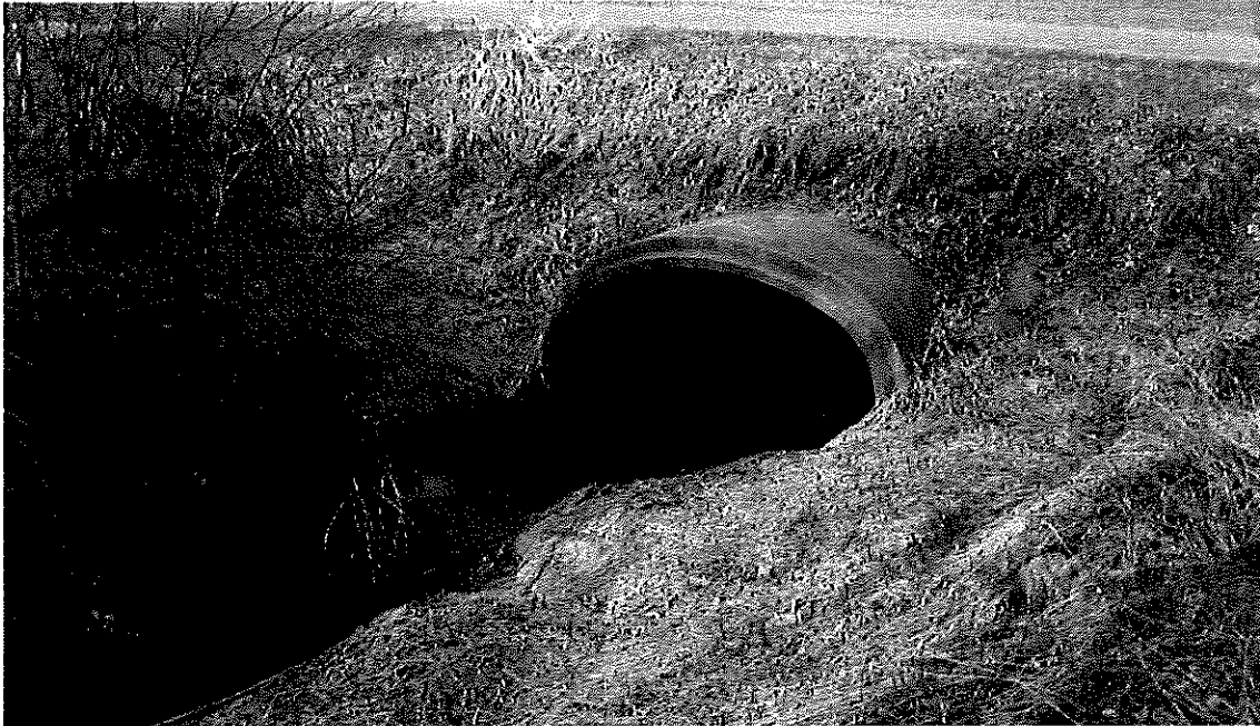
Picture No. 15 shows the downstream eastern end of the 5-foot by 9-foot elliptical RCP culvert crossing under East Paris Ave. Picture is taken looking southwest.
