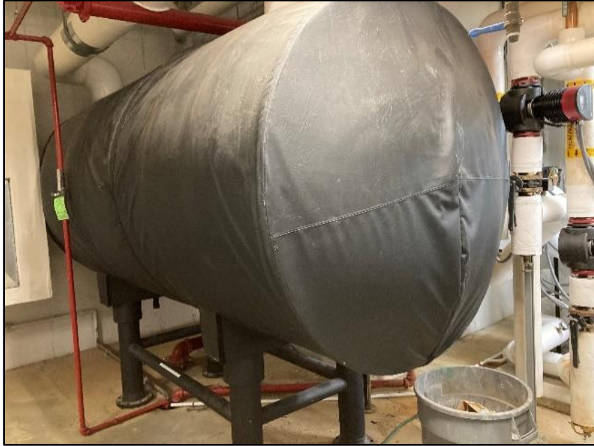
Chilled Water Storage Tank
