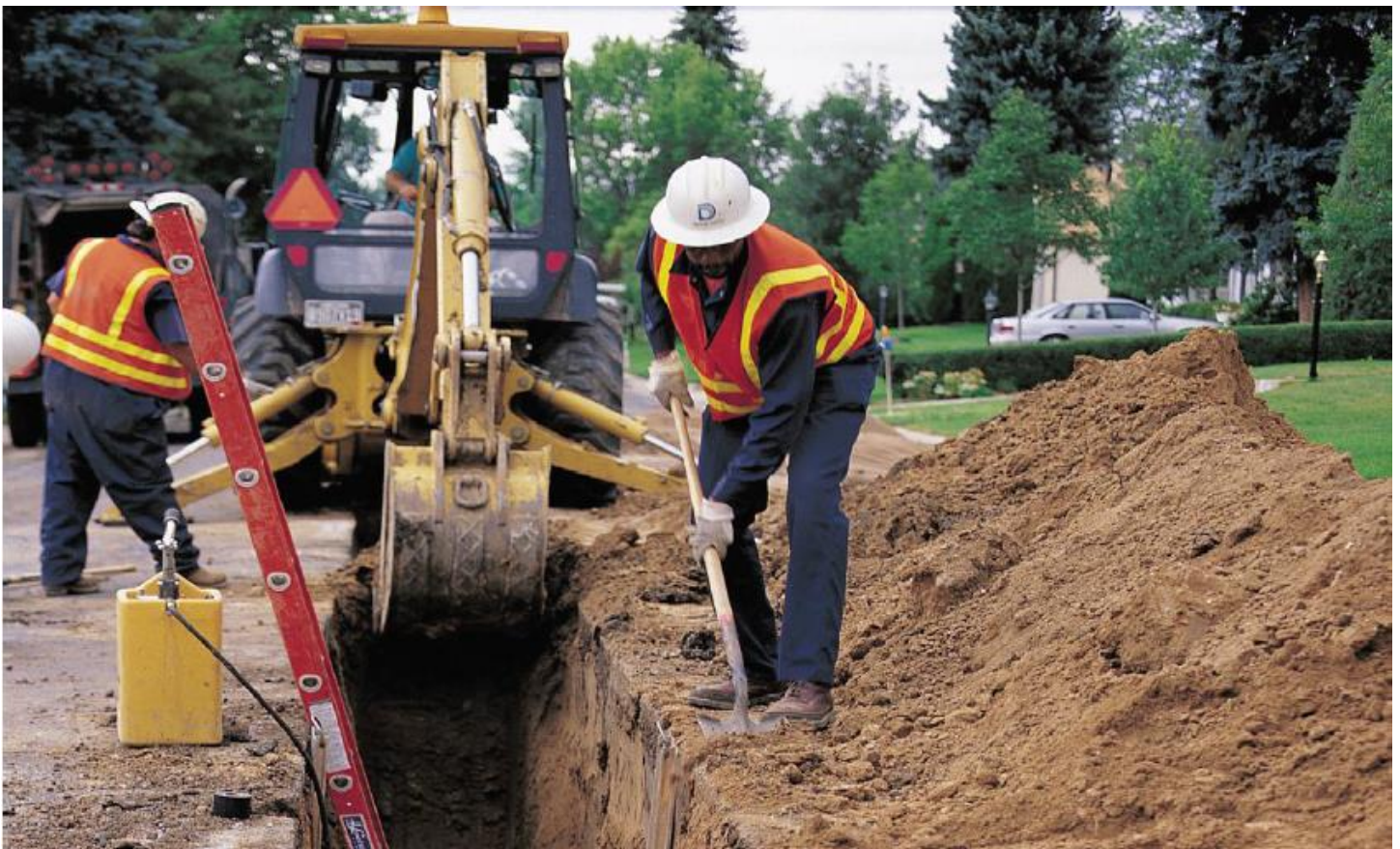
Residents may soon see construction work like this taking place on Lincoln Road, 29 th Street and Jeffrey Drive to connect 4 homes to the public water supply.
