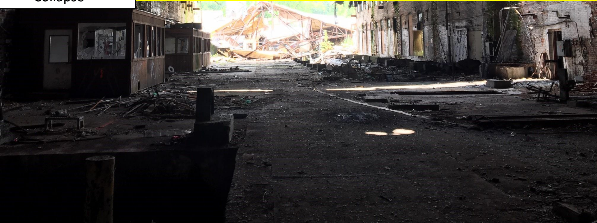
Area of Imminent Collapse
