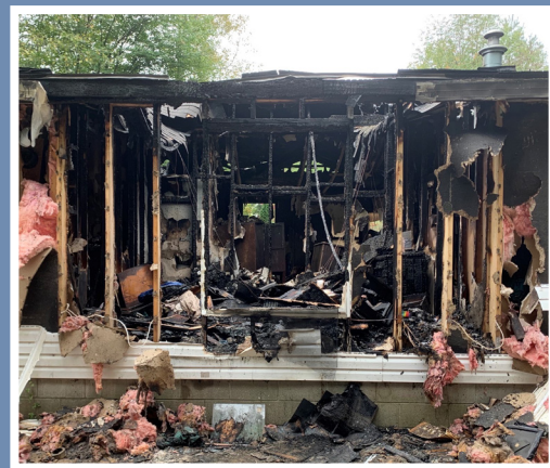
Exterior of the Stille residence after the blaze on October 1.
