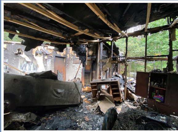
The Stille residence after the home was engulfed by flames on October 1.
