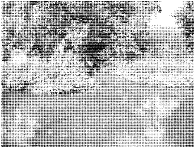
A view looking west at the road side ditch as it outlets into the North Branch of the Macatawa River.
